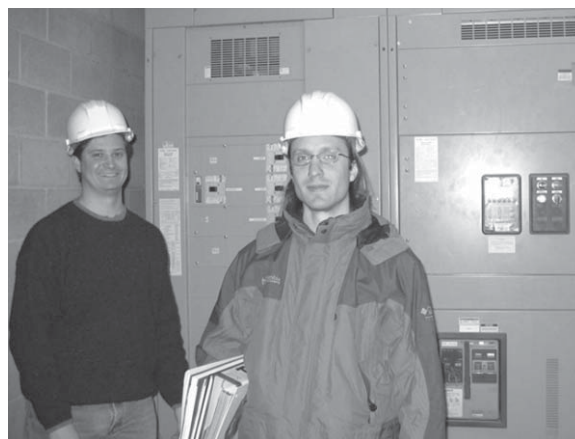
John and Andy visit the electrical power switching room in the basement of the CIC building to check out where the circuit breakers for the data center would be installed.
