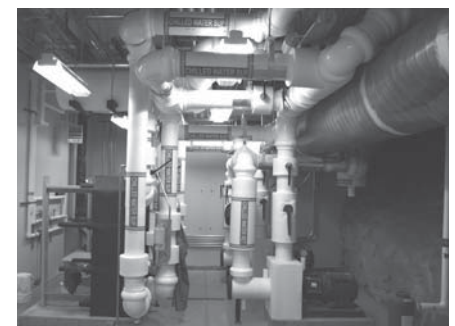
Piping, redundant pumps and heat exchangers that provide chilled water to the DCO.
