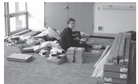
Michael Stroucken begins assembly of the DCO computer storage racks.
